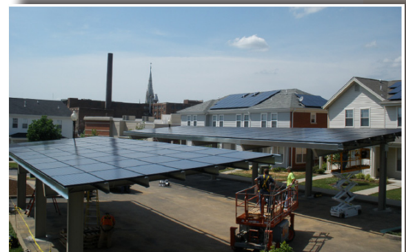
Photo: Courtesy of Nick Cohon of Real Goods Solar Workers installed solar panels on roofs and carports at Renaissance Place in St. Louis, Mo.
