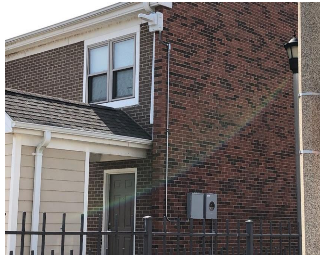
LaSalle Park Site Security Cameras
