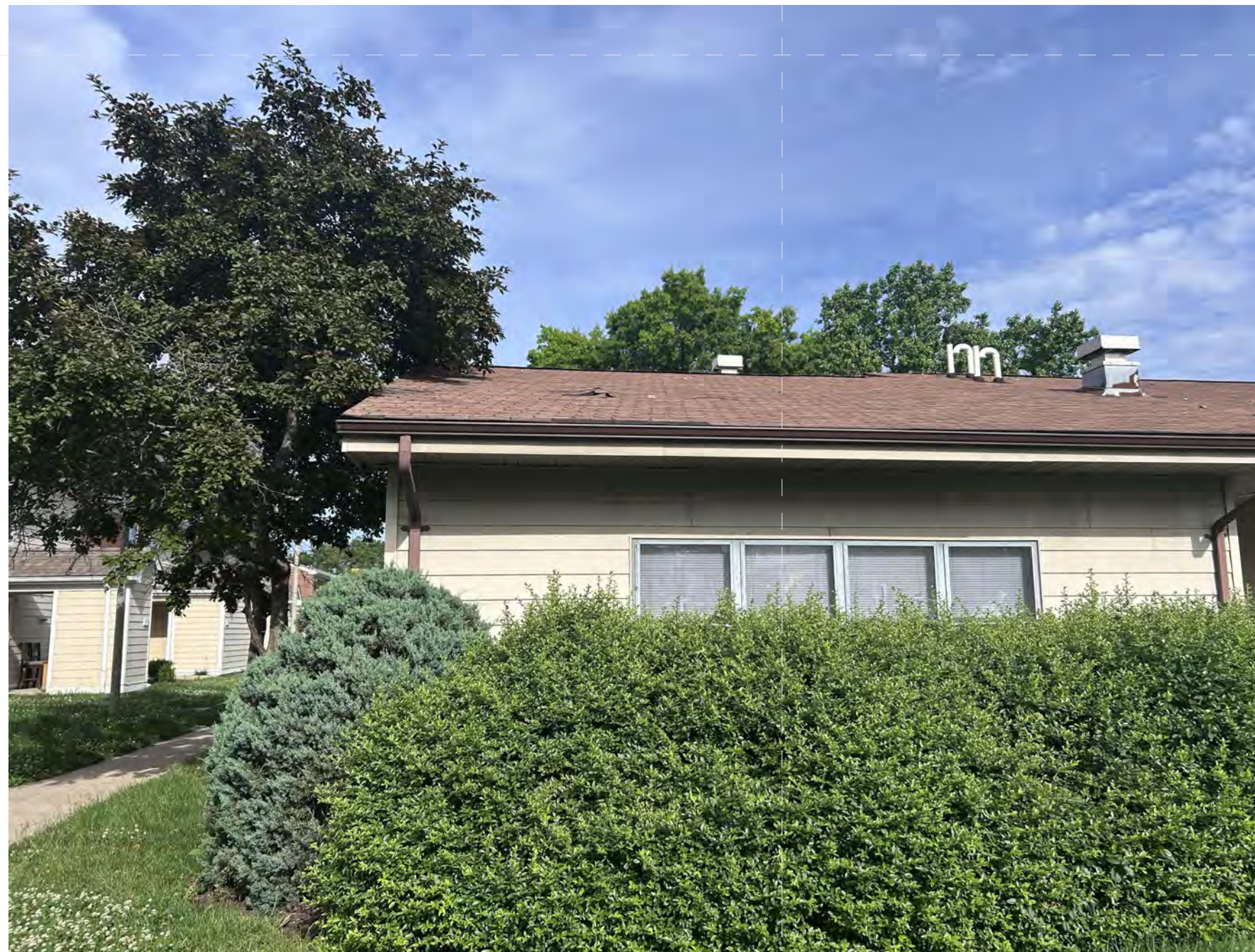
A3 LOOKING EAST AT WEST FACADE - SUBSTRATE DAMAGE, AND EXISTING ROOF PENETRATIONS TO REMAIN 1/2" = 1'-0"
